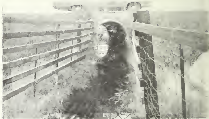
SOUTH ENTRANCE Note water in stockpass
